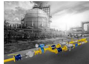
Gas control systems
