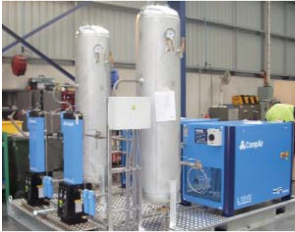
APA Gasnet Compressor Skid
