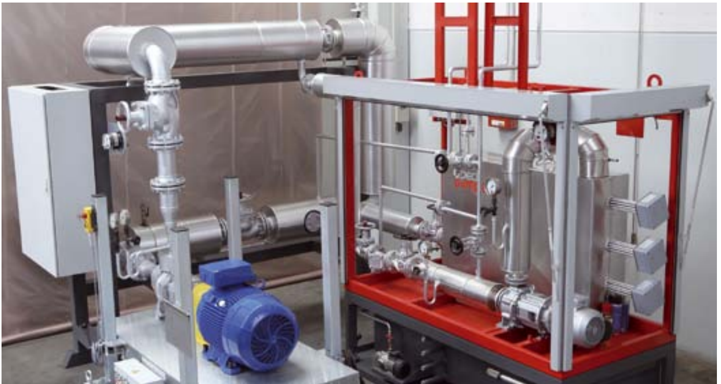
Thermal oil test stand with pump surveillance system on the premises of Speck in Roth.
