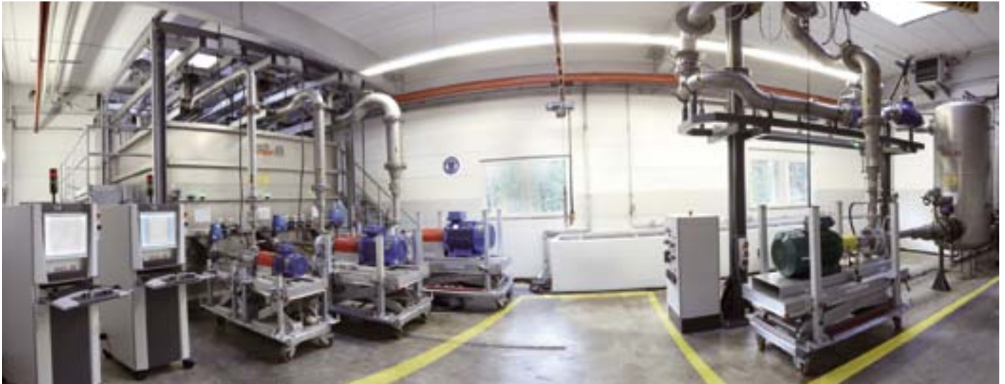
Computer-controlled and fully automated test stands on the premises of Speck in Roth.
