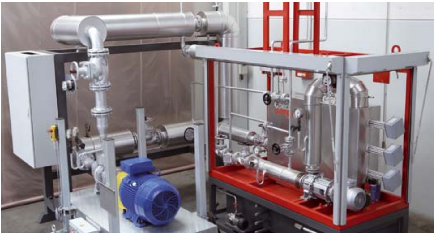
Thermal oil test stand with pump surveillance system on the premises of Speck in Roth. Research of impacts of high temperatures up to 350 °C on the lifetime of the pumps.
